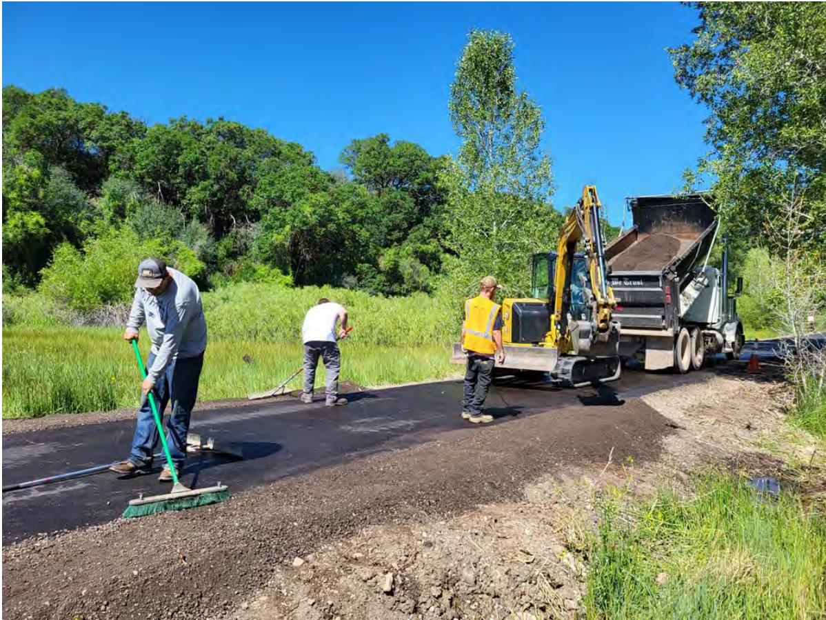
Photo – The Holmes Excavation crew rebuilding the shoulders (very carefully) after the asphalt has been replaced
